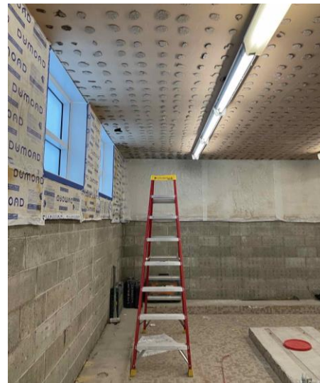
Stormonth: Locker room demolition has begun, this space will be repurposed into an additional classroom.
