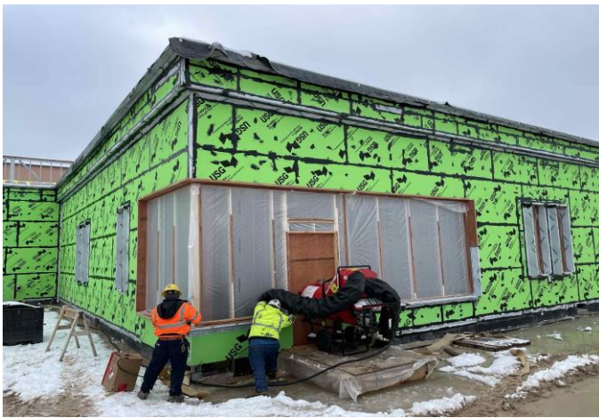
Bayside: Prepping the exterior for air barrier install at the new district office
